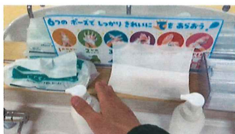
Fig. 6: Example of improper paper towel installation.
